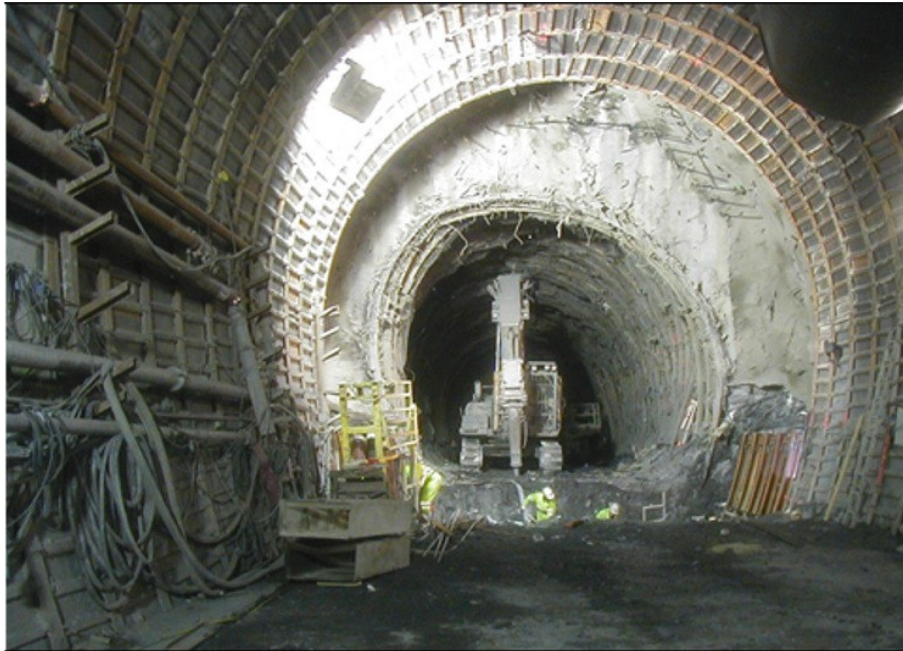
Figure 1 Squeezing rock reduces the tunnel cross section. This is shown dramatically in this photograph taken at the Saint Martin La Porte access tunnel along the Lyon-Turin Base tunnel, where re-profiling of the highly deformed cross section took place.
