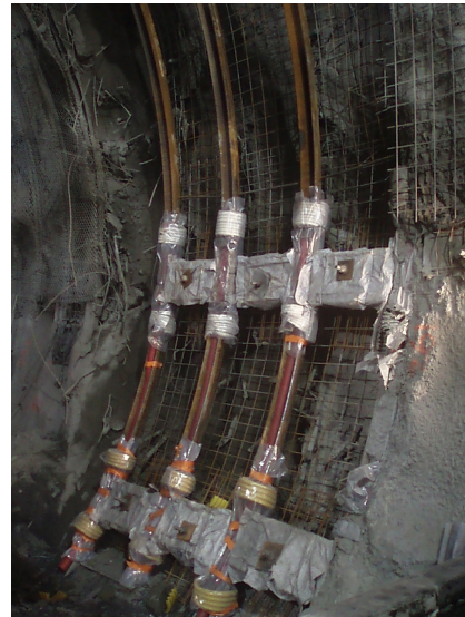
Figure 7 Yielding support with Hidcon elements incorporated in the shotcrete lining and between steel sets with yielding couplings. Installation details as adopted in the Saint Martin La Porte access tunnel.
