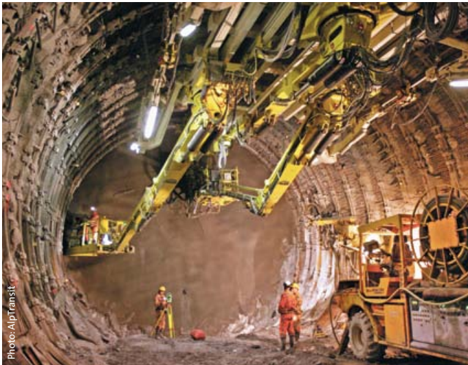
A world's first in tunnel construction at great depth: flexible steel arches control the huge mountain pressure.
