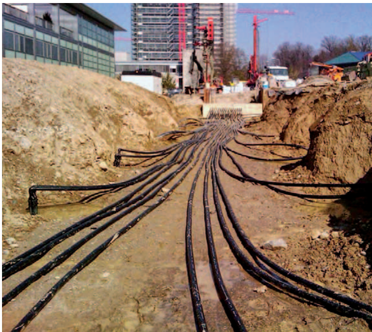
A model concept on ETH Zurich's Campus Science City: In summer, heat lost from buildings is stored by way of 800 earth probes in the ground to be re-used as heating in winter.
